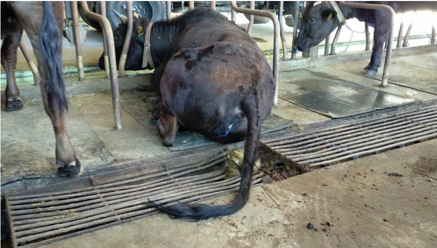
A cow lying on the damaged and gapped grating, unable to stretch, as a result has to wrench its body
